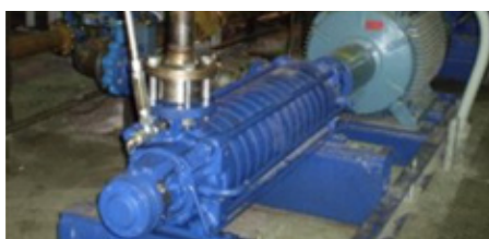
Low pressure pumps
